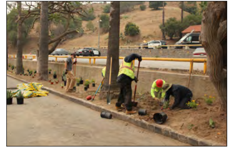
WATER CONSERVATION was evident by the drought-tolerant and native plants installed by crews from several SFV member companies. A big thank you to crew members and their companies.
